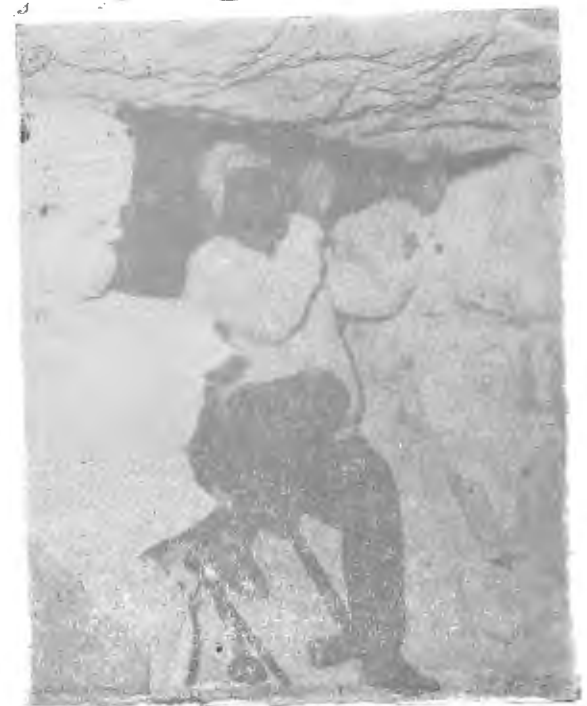
— Mr. Mohammed widening the open between the main Library and its exten- sion.
